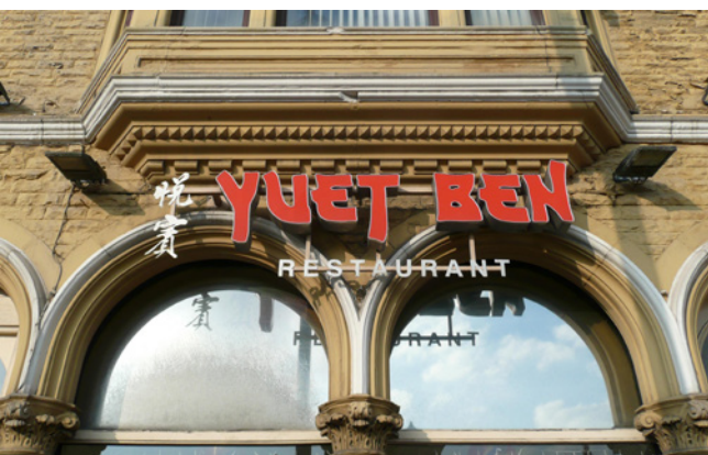
1873,3. The nail-head decoration on the stonework supporting the oriel window (compare the dog-tooth decoration on the mullions on Oriel Chambers, e.g. Footsteps, pp. 206-207) and a glimpse of the foliage capitals. GHJ.
