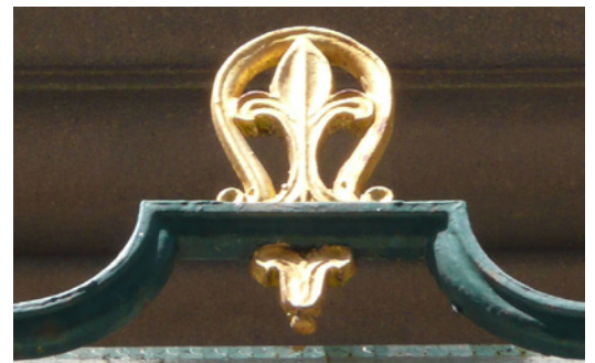
1864,27 and 28. The three fleur-de-lys decorations on one of the window frames at Oriel Chambers. Before WWII bombing destroyed part of the Covent Garden façade there were more than 200 and, if you are keen enough to go there and count them, there are still 168. GHJ.
