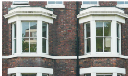
1864,22. First floor bay windows at nos. 20 and 22 Catharine Street in 2014, part of the terrace undergoing renovation between Falkner Street and Upper Hope Place. GHJ.
