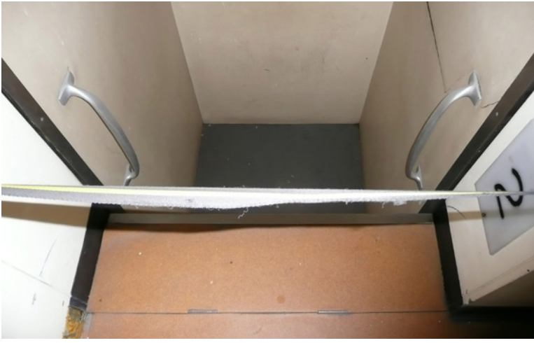
2013,3. A view of a compartment as it approached floor 2 with the taped barrier in position.
